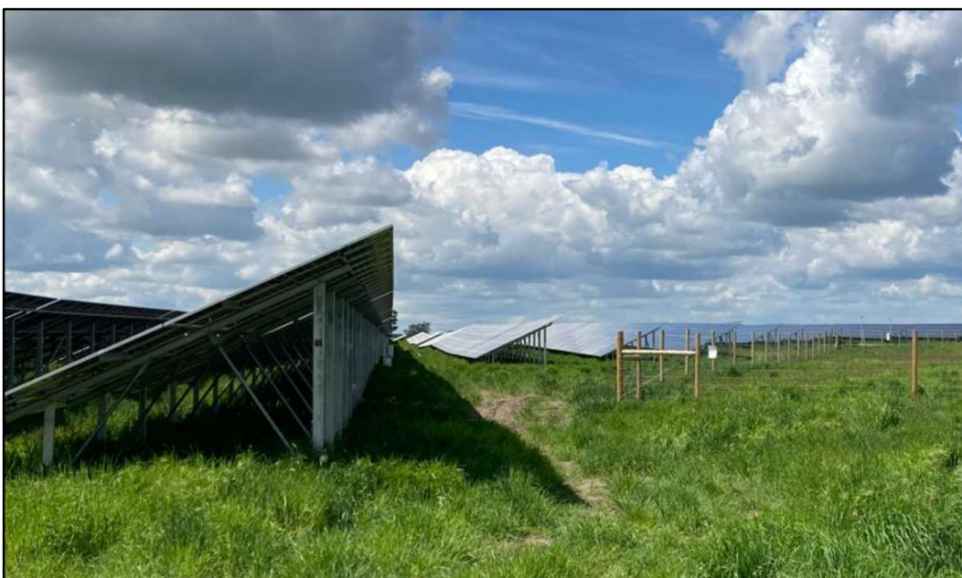
Plate 3.2 Example of a typical mounting structure
