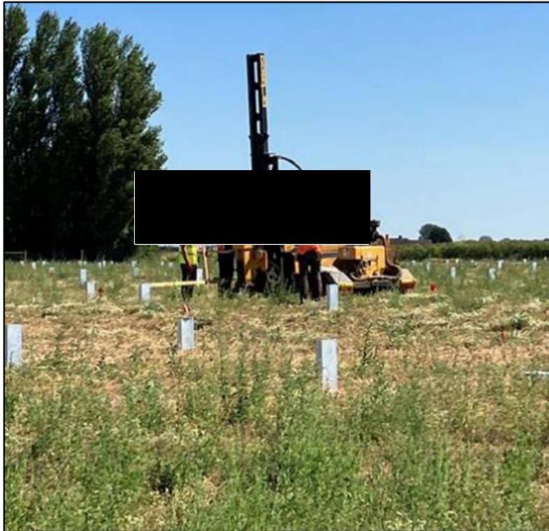
Plate 3.14: Example construction piling for the installation of the Solar PV mounting structures
