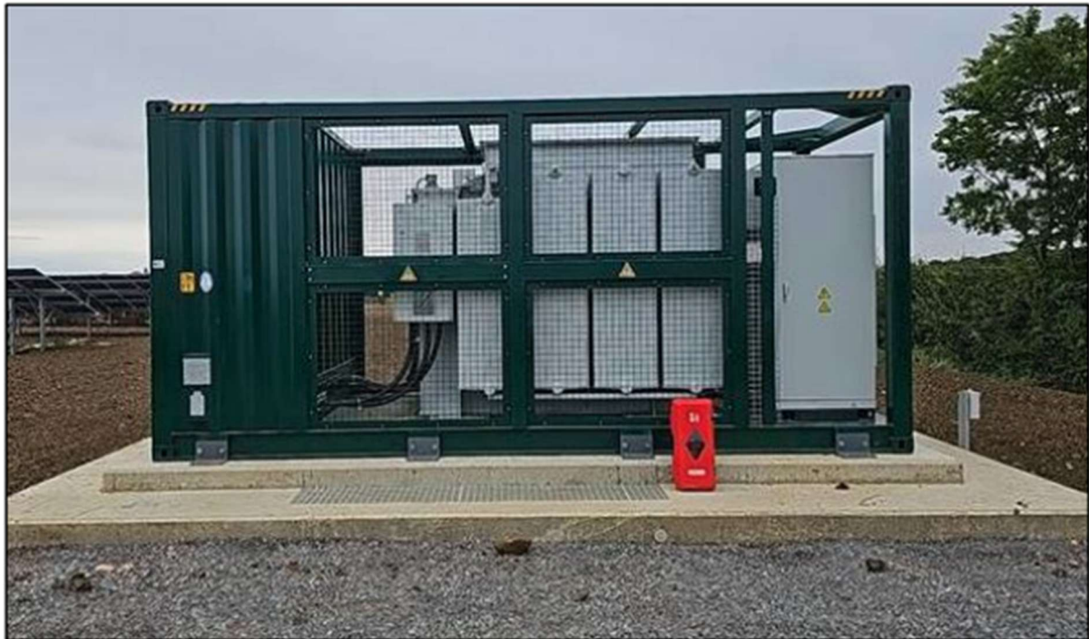
Plate 3.8 Typical Inverter Transformer Station
