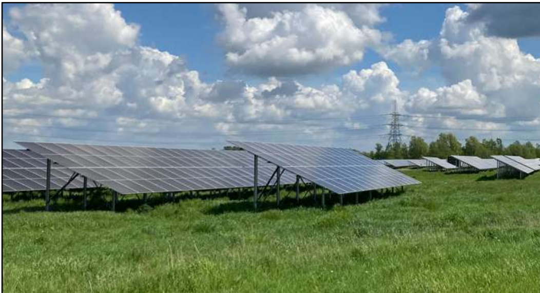
Plate 3.1 Example of a Solar PV module and mounting structure
