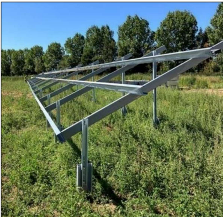
Plate 3.13: Example Solar PV mounting structure
